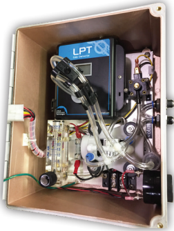
Inside of the DCC-SD showing an LPT-A gas detector mounted inside the enclosure.
